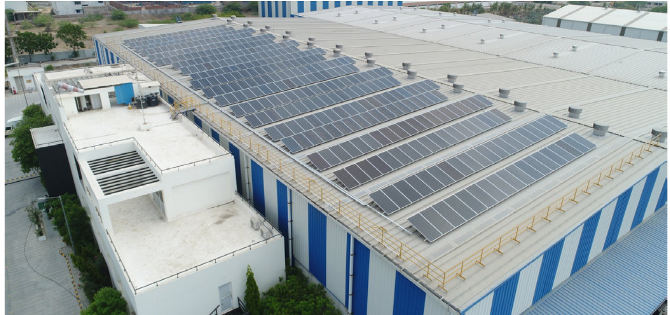
150 kW rooftop solar power plant installed at our manufacturing facility in Ahmedabad, India.
